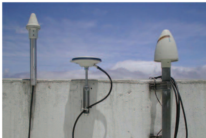
Figure 6. GPS antennas installed on the roof of a calibration laboratory.
